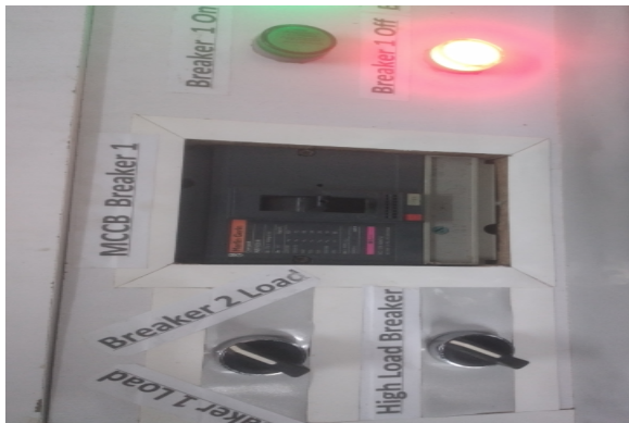
Fig. 6: Shows the breaker # 1 is off
